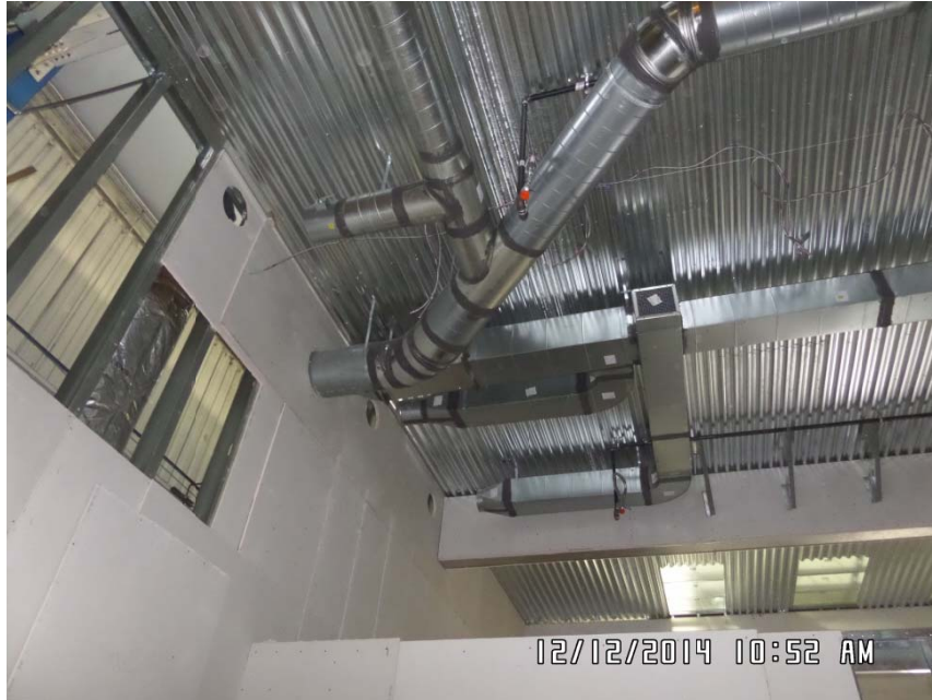
Overhead Ductwork at Courtroom Mockup
