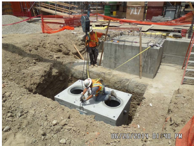
Sand-Oil Interceptor Tank
