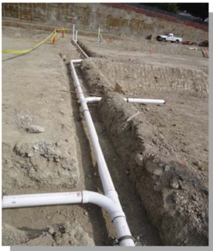
Underground Wastewater Line
