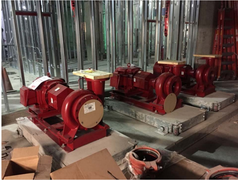
Condenser Water Pumps
