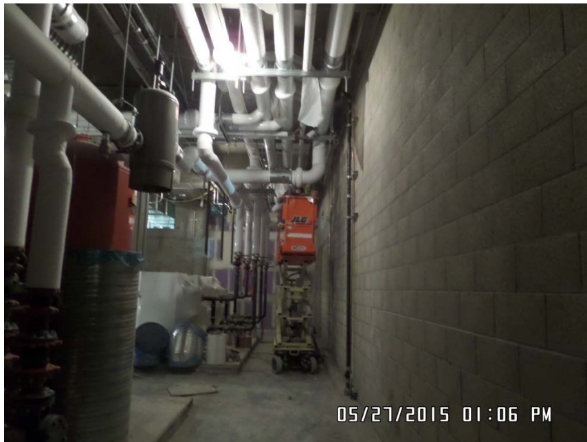
Piping Insulation in Basement
